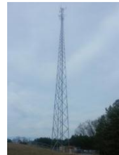
One of seven wireless towers in Columbia County that provides enhanced communications capabilities for local public safety entities.
