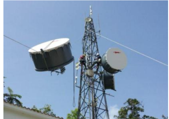
Two workers install broadband equipment in Cayey, Puerto Rico, to increase Internet capacity and support an electronic health exchange.
